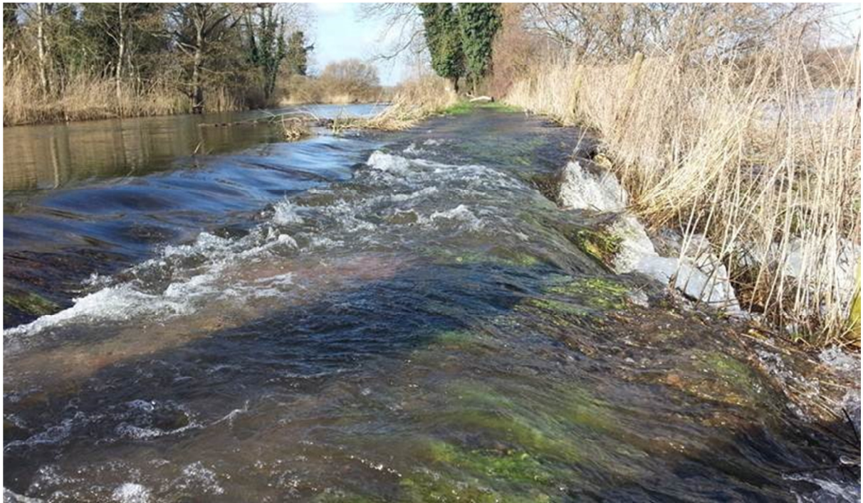
Figure 3: Flood Damage and Overtopping, Burghfield
